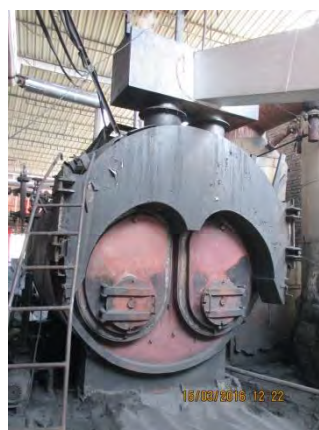
Caption: Boiler unit at Vijay Anand
